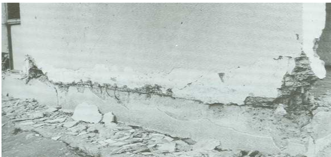
Fig 11: Failure of shear wall observed after Chilean Earthquake 1985 (Wyllie et al. 1986).
